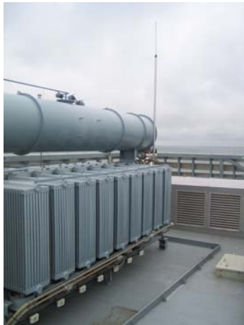
Fig. 11 Cooler System on Roof
